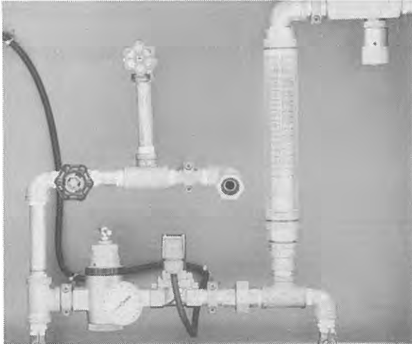
Water Meter Control
